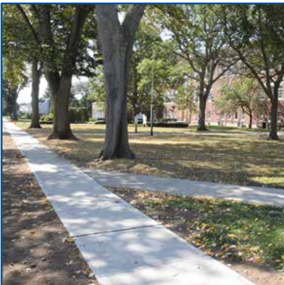
Site work to repair sidewalks and curbing, among other infrastructure, was performed at various schools.
